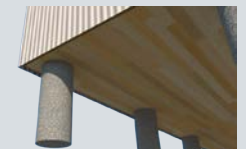
The structure rests on poured concrete pilings that protect it from flooding and encourage ventilation
